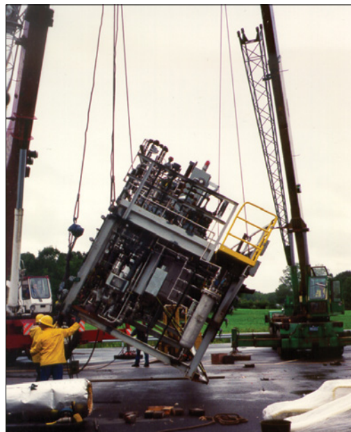
FIGURE 1. The owner can opt to completely contract out the comprehensive design and construction of the pilot plant, but this option assumes a great deal of trust in the chosen contractor's skills
